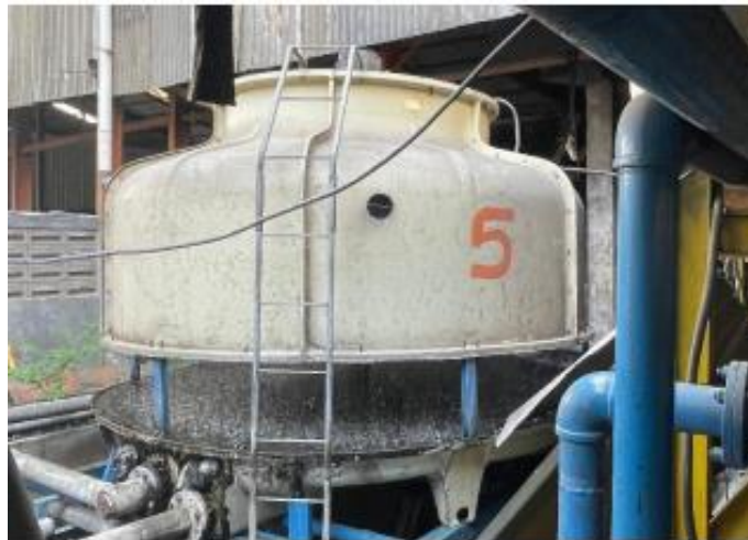
Gambar 6. Coolong tower D
