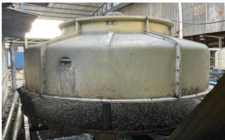
Gambar 5. Cooling tower C
