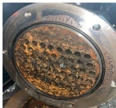
Gambar 3. Seal Di Oil Cooler
